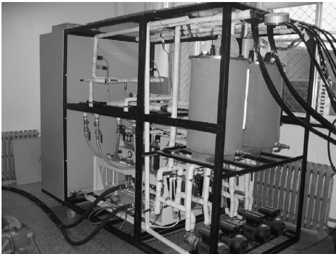
Fig. 7. Cooling system plant for the beam pipe.
